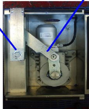
Underground Motor In Chamber
